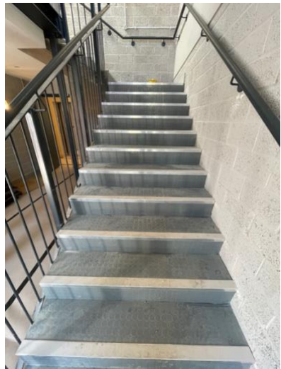
Staircase in Parfitt finished to substandard level!
