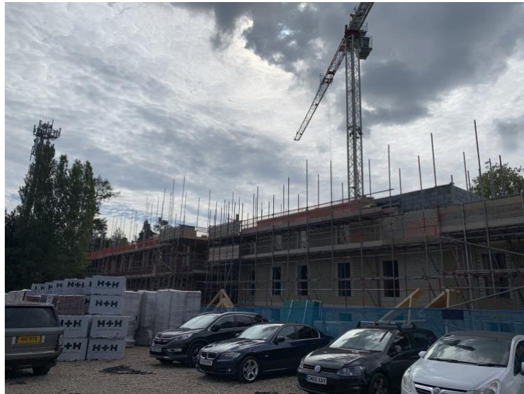
Contractor's car park area now in use for its proper uses – almost!
