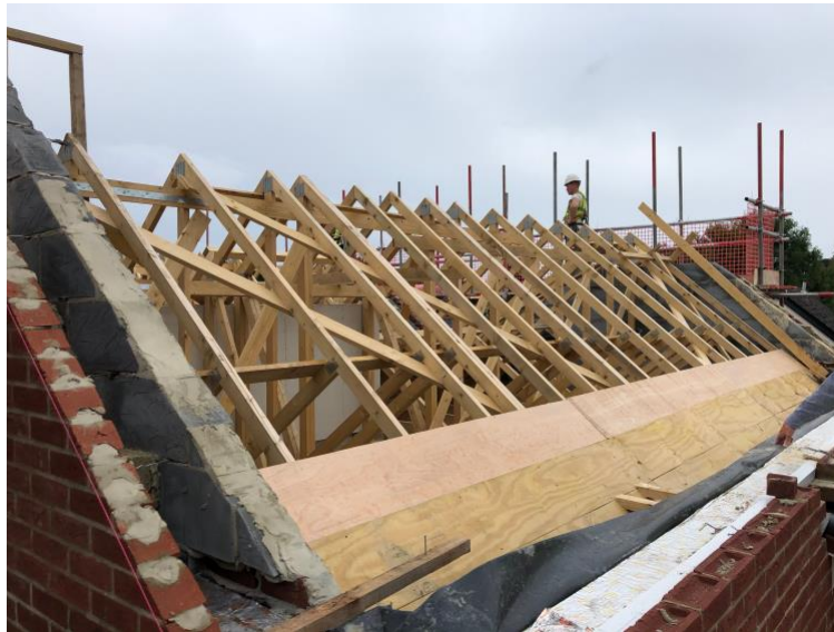
Finishing the roof on Parfitt ready for fixing felt and battens next week
