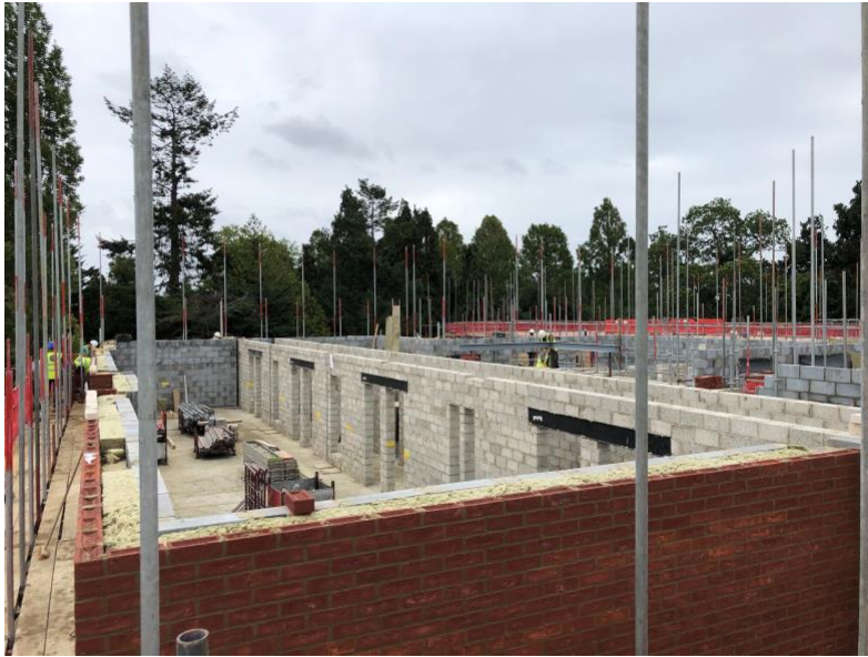
Townsend is ready for the 3 rd floor to be installed next week
