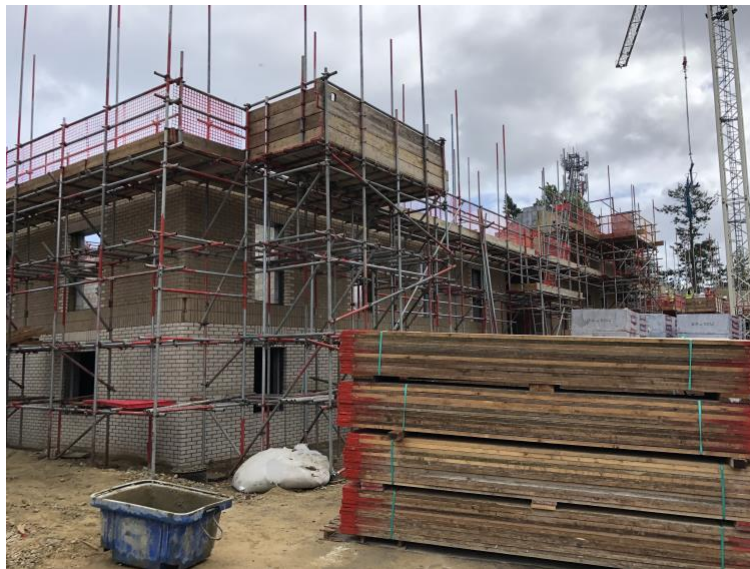
View looking at Preddy which is now almost ready for the roof trusses to be installed
