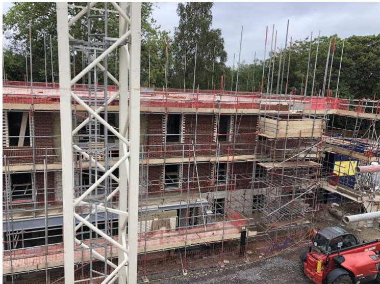
View of MacDonald from Preddy's top floor with last floor slab in place
